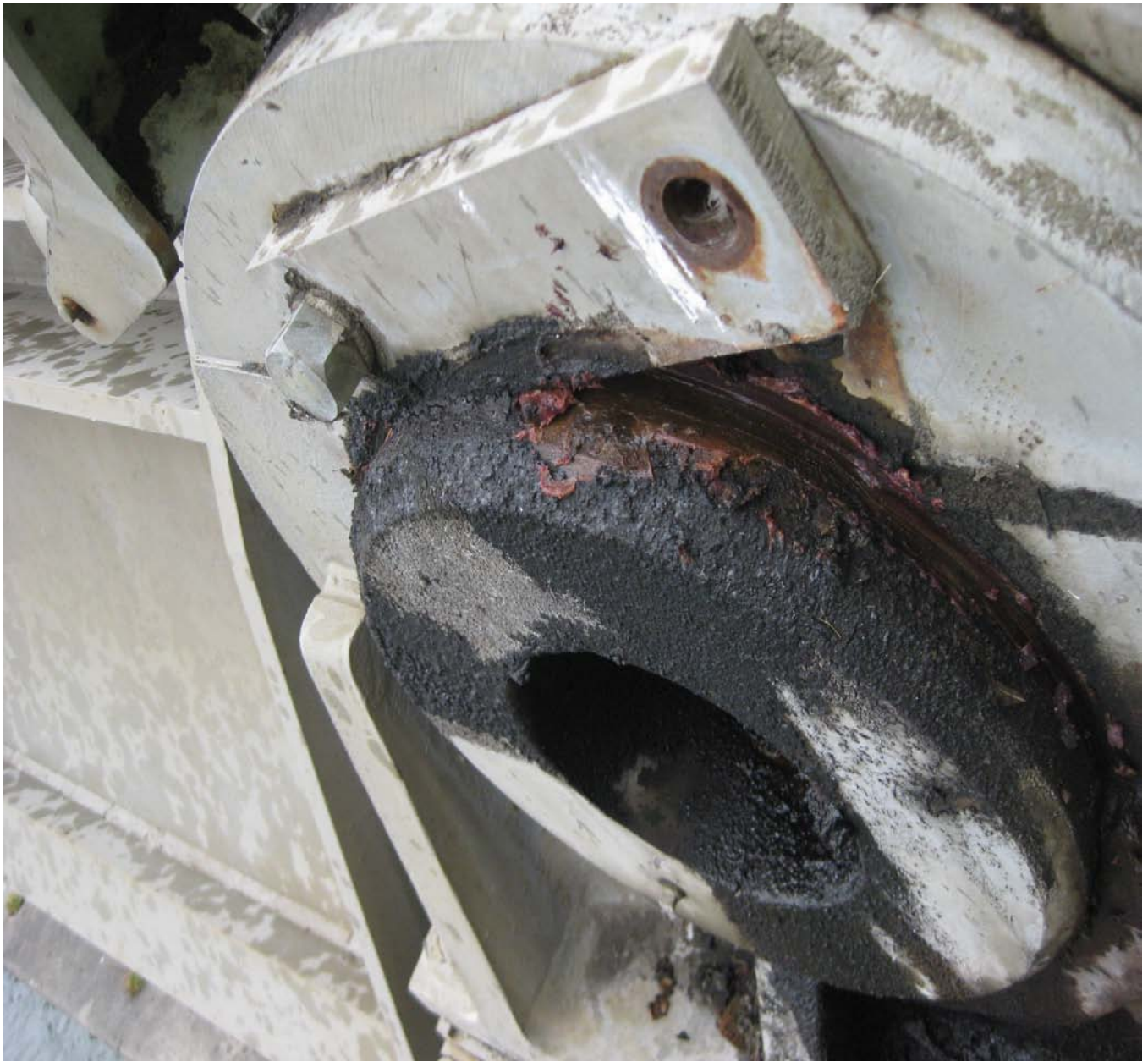
Spillgate 9 seized trunnion pin. Gate tagged out of service.
